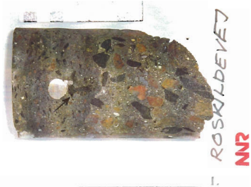
Figure 3.10 Core taken from a shotcrete repair of a sidebeam at a bridge. The arrow behind the reinforcement bar indicates air void and bad compaction due to poor workmanship. This will reduce the durability of corrosion protection of the reinforcement bar.
