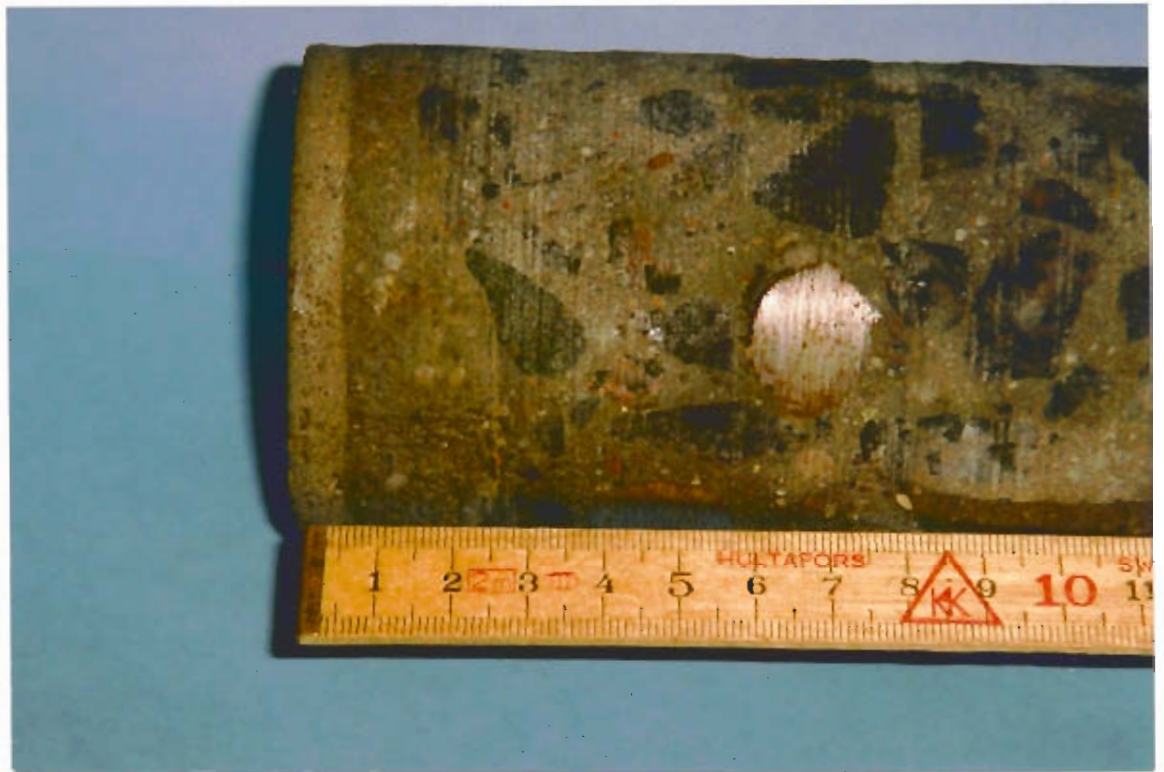
Figure 3.8: Core drilled out of a repair with mortar and shotcrete. The mortar has been applied as a finishing layer on top of the shotcrete. The casting joints between the different materials are filled out fully and the materials are well compacted and homogeneous.
