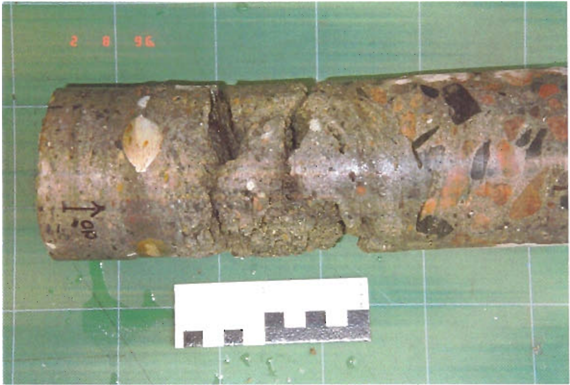
Figure 3.12 Core taken from repairs made with shotcrete. The shotcrete is poorly compacted and there are large air voids in the repair materials. This reduces the durability of the structure.
