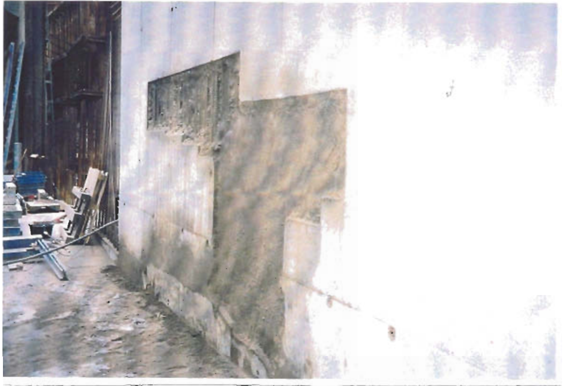
Figure 3.4: Repairs made with shotcrete after the first layer was applied. The area around the repair framed in order to avoid shootcrete on the surrounding surfaces.
