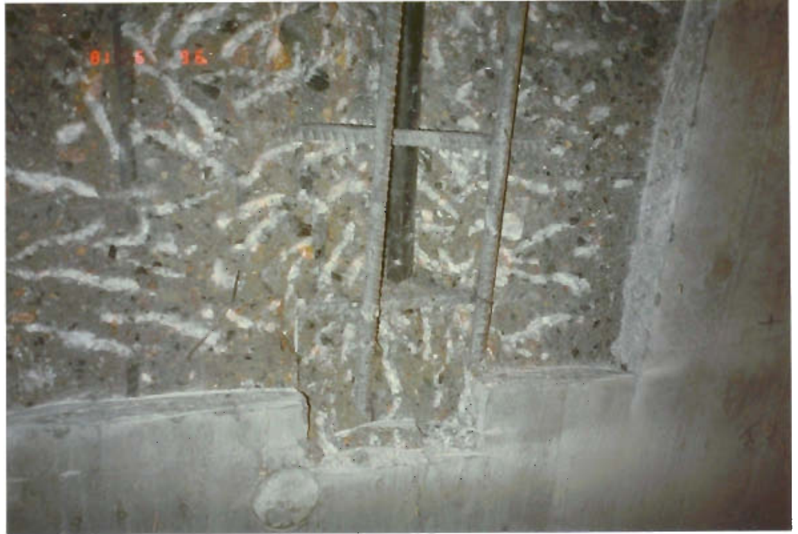
Figure 3.1: Removal of defect concrete. The concrete was damaged by frost expansion of the black cooling pipe behind the reinforcement. Damaged concrete was removed by cutting with pneumatic handheld hammers and the edges of the repair was cut with a diamond saw at an angle of 90° to the surface. Where reinforcement was exposed the concrete is removed min. 20 mm behind the bars, in order to admit materials to surround the reinforcement sufficiently.
