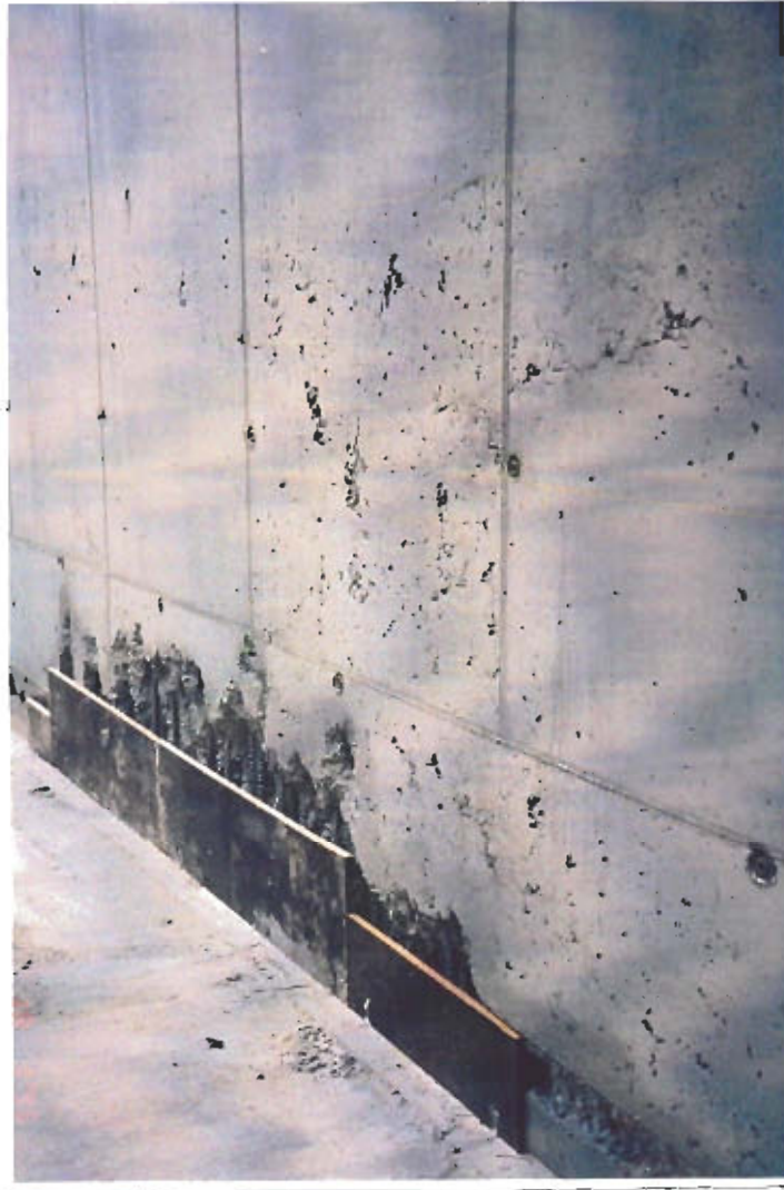
Figure 3.3: Filling out the hole in the lowest part of a wall in a tunnel with repair concrete. The hole in the wall was caused by lack of removal of ice before casting. The formwork for the repair concrete should be higher than the repair. The defect concrete above the repair should be removed before starting the repair process.
