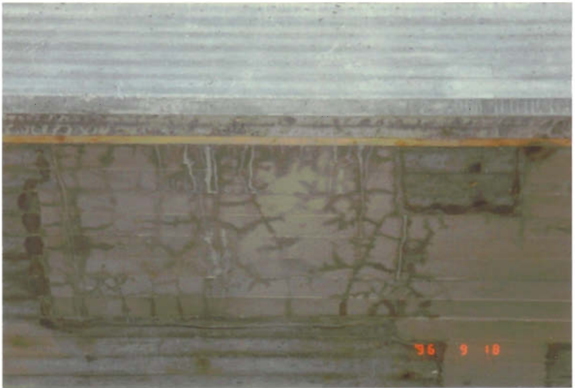
Figure 3.6: Repair with mortar. The surface cracked because of lack of protection against evaporation. The repair should be protected against evaporation for instance by attaching plastic.
