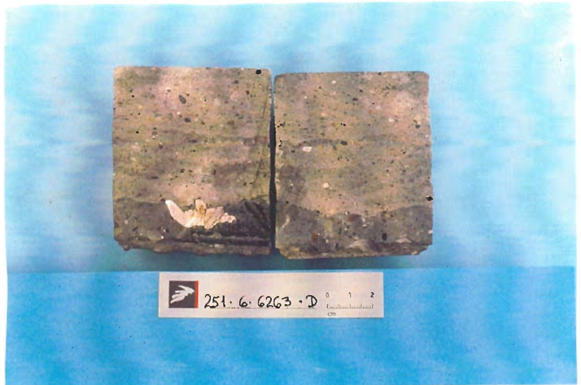
Figure 3.9 Core taken from a repaired tunnel wall made with shotcrete. The layer of the spraying is visible. The repaired is homogeneous without defects and there is full adhesion in the casting joint.
