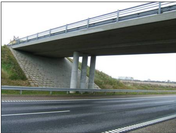
Figure 1. Image showing part of the west side of the bridge. On the edge beam is seen a colour difference between two types of concrete. The three columns are cast with different concrete types.
