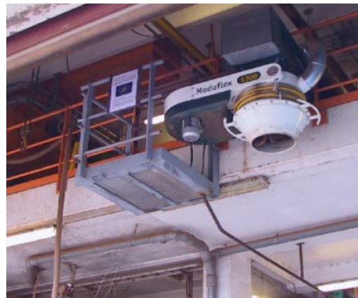
New bio ash outlet at Lynetten WWTP
