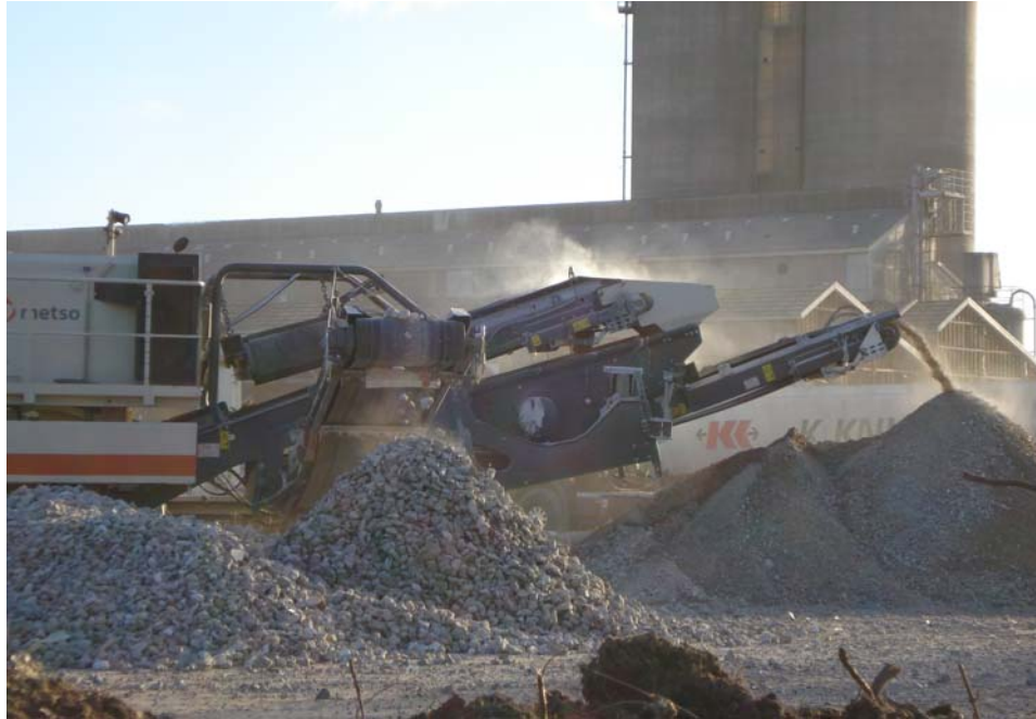
Figure 1. Mobile crusher sorting concrete rubble into fractions to be used for road construction and back-filling purposes.
