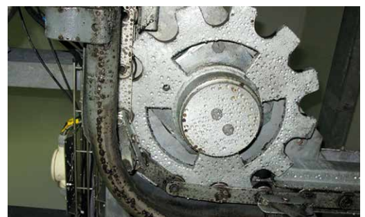
Conveyor structure dripping
