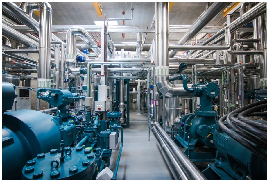
Figure 1: 5 MW thermal heat pump system for district heating in Copenhagen [Source: HOFOR].
